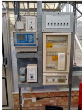
Typical Glasshouse compartment with adjacent Climate Controls controller.
