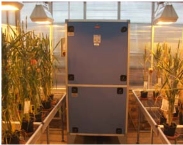
Air conditioned compartment from G31. Note polycarbonate cladding and air conditioning unit
