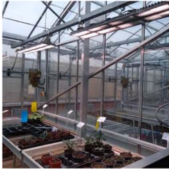
Compartment in G34, naturally ventilated, showing Kropstek 400 watt LED lamps
